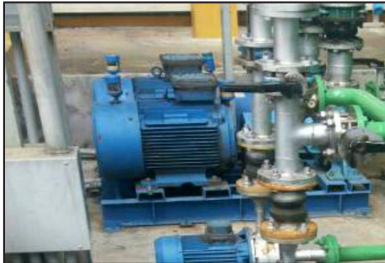
Over greasing led to frequent bearing failure.
